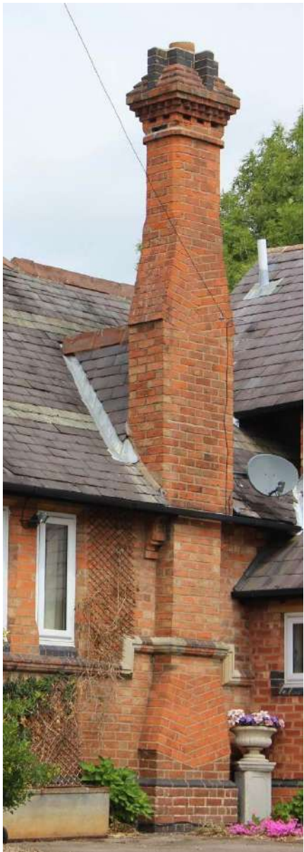
The heavily moulded and prominent chimneystack at the former Old National School.
