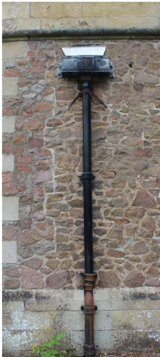
The cast iron downpipe with a stamped hopper at St Mary's Church.
