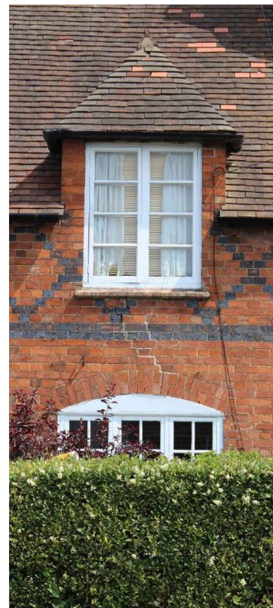
Right: Original timber casements and good replacements of the original units (timber framed or matching design) are the most common windows throughout the Conservation Area.
