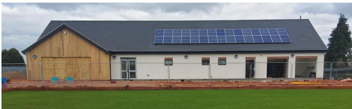
Solar PV installation on the Shakespeare Park Pavilion
